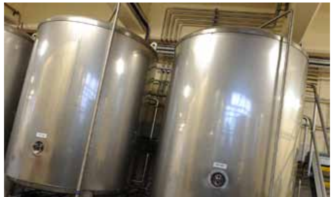
We also bought 3 X 20 brl enclosed fermenters and assembled the plant upstairs in the redundant old cask washing area, conveniently located behind the bottling tanks. Cooling water is supplied from a stand-alone chiller unit.
