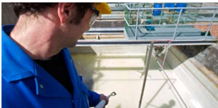
Safety dump pit with fire wall
